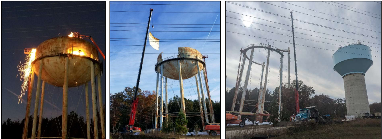
Photos show the progression of the demolition and dismantling of old water tower
