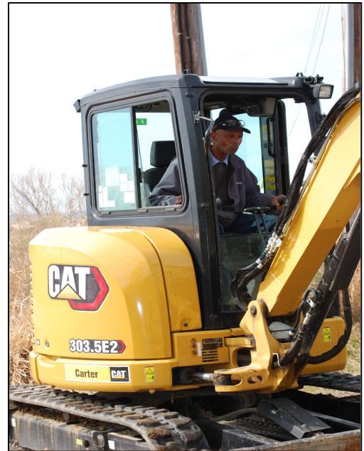
Pictured above is one of our Construction staff responding to an emergency waterline repair.
