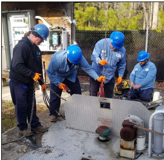
Pictured above are Maintenance staff preparing to remove and repair a pump.
