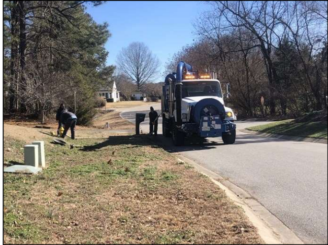
Pictured above are maintenance and collections staff responding to a reported sewer back up. Maintenance and Collections personnel are on call and available 24 hours a day, 7 days a week, 365 days a year.
