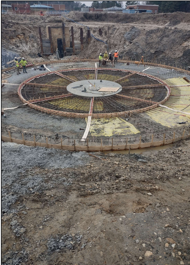
Photo shows construction work on Secondary Clarifier #1 at the Marlay-Taylor Water Reclamation Facility.
