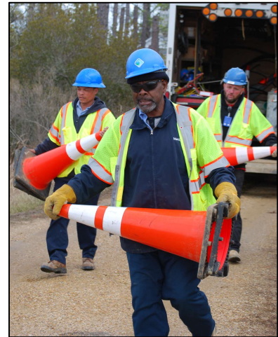
Water lines break at all hours of the day and night. MetCom's staff has to respond quickly to maintain service to our customers.
