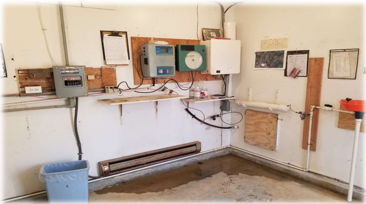
Inside of Town Creek # 6 WPS
